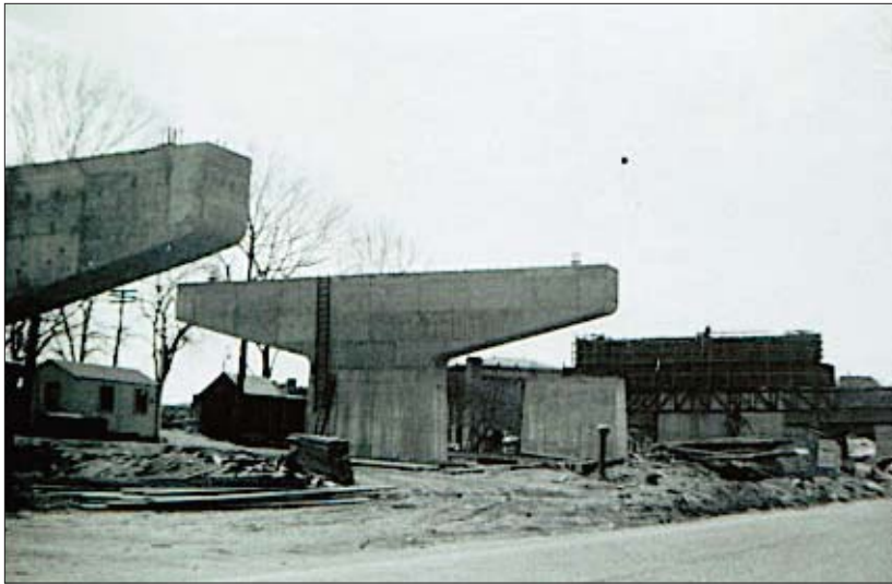
Construction of the Casey Overpass in 1952 - 1953. Jamaica Plain Historical Society Photo Gallery. Ed Barrett photograph.
